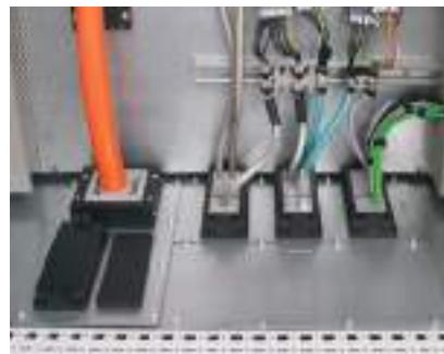
Cable routing via module plates in the base of a Rittal TS8 enclosure. Mounting with icotek gland plate KDR BMP.
